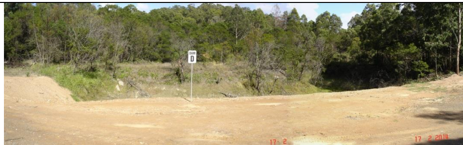
Dam D - Vegetated sediment dam with the dam wall to be raised 2m to increase the capacity to 25ML. Total capacity still available for collection of runoff water after the February 2014 rain event.
