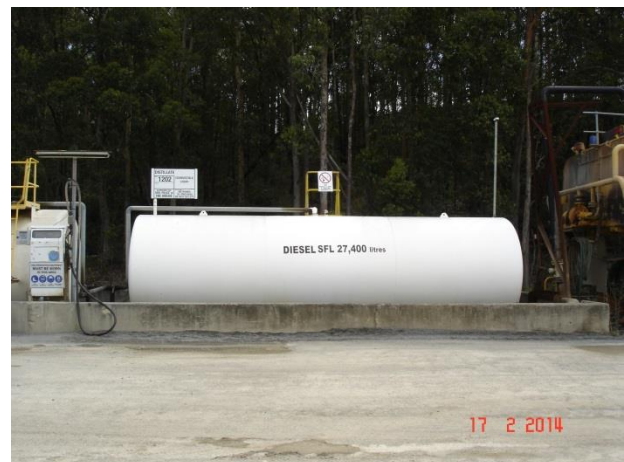
Bunded diesel tank adjacent to the waste oil and grease storage area.
