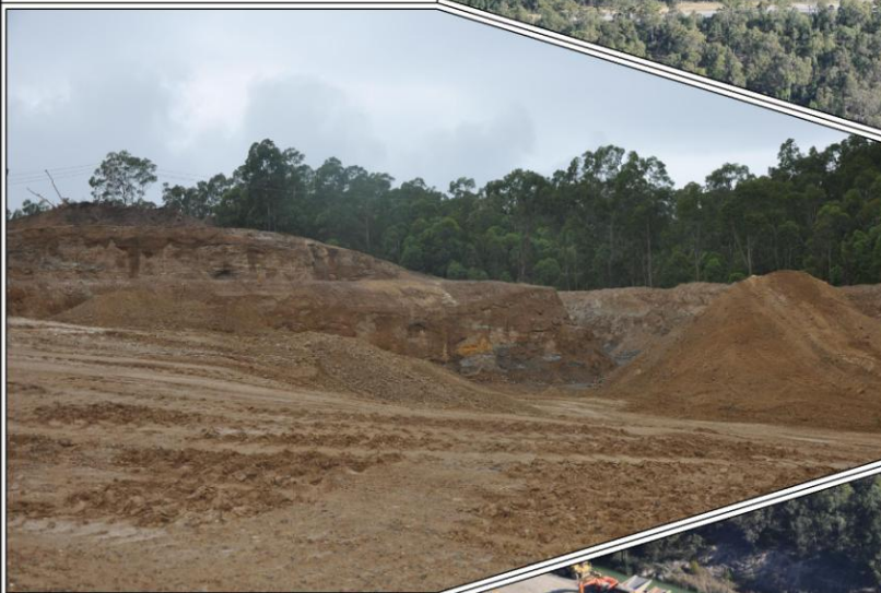
Plate 1.3: A view to the southeast towards the active area of the existing Mid Pit Extraction Area (Ref: E559T/048)
